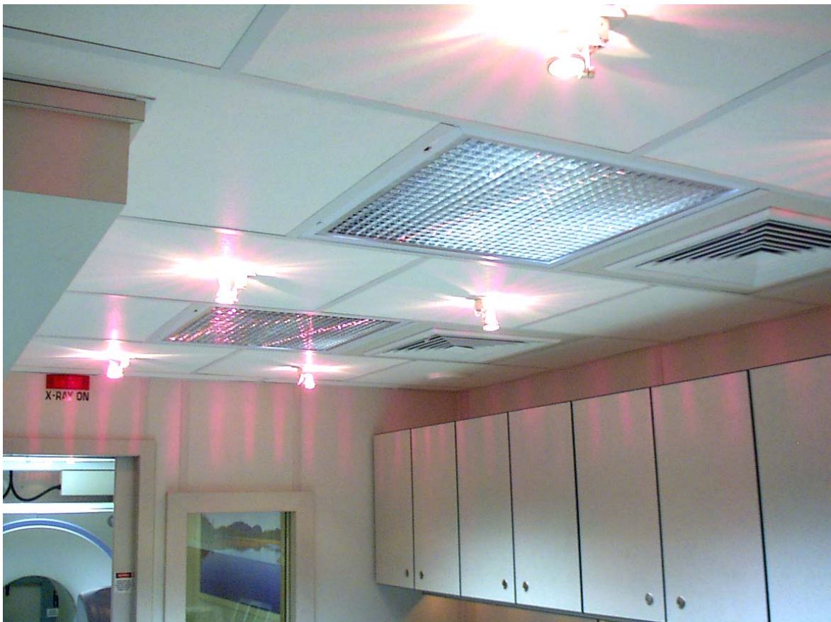
Figure 50: Control Room Overall Lighting
