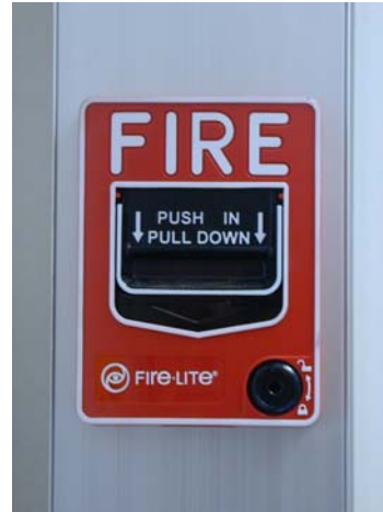
Figure 20: Fire Alarm Pull Station
