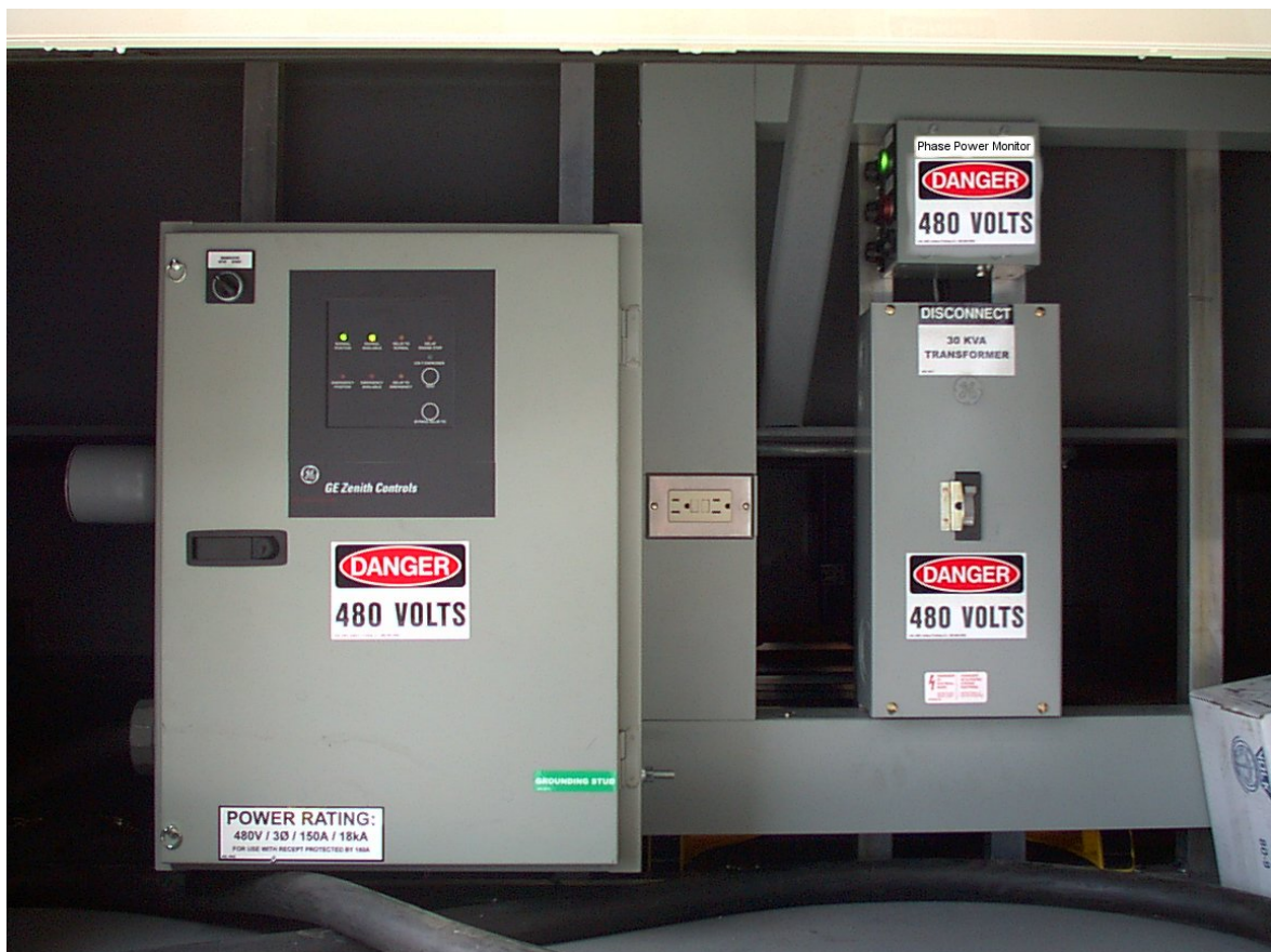
Figure 30: 480V AC ATS and Phase Power Monitor
