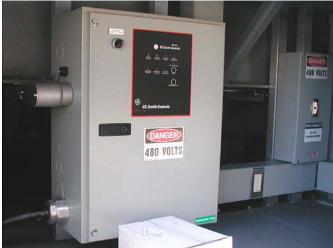
Figure 25: Automatic Transfer Switch
