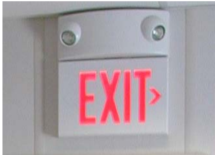
Figure 16: Control Room Emergency Lighting
