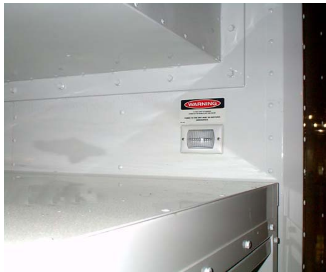
Figure 53: AC Power Loss Strobe Light
