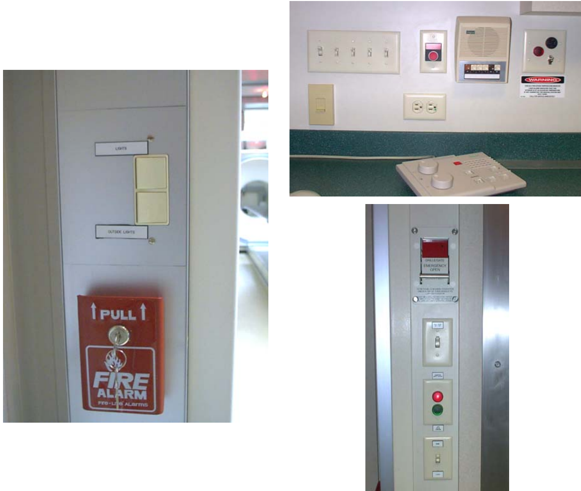
Figure: 11 Mobile Unit Controls
