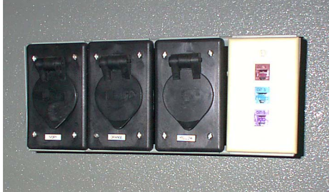
Figure: 12: Phone & Data Line Connections
