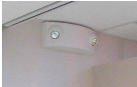
Gantry Room Emergency Light
