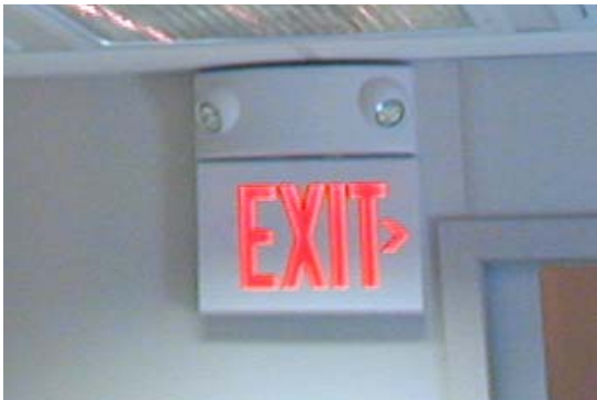
Control Room Emergency Light
