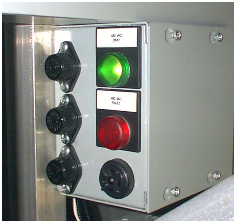
Figure 31: 480V AC Phase Power Monitor
