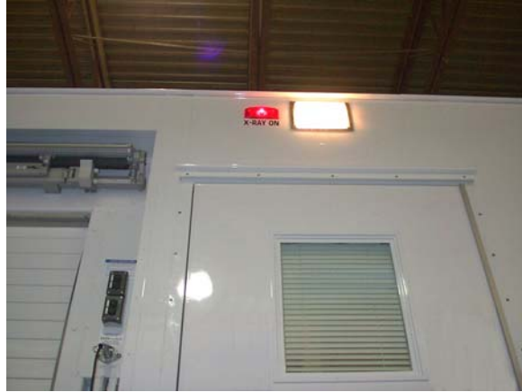
Figure 49: Staff Door Lighting
