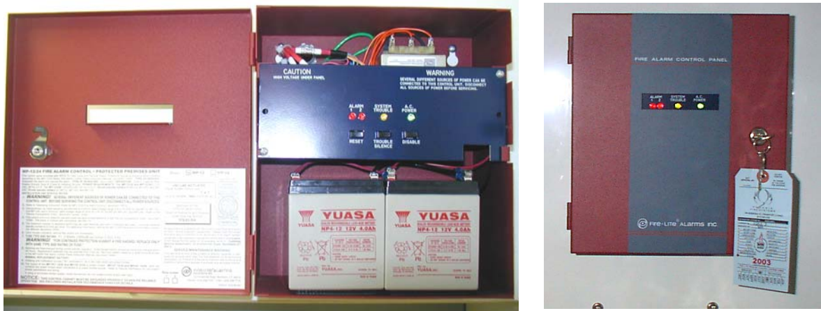
Figure 19: Fire Alarm Control Panel
