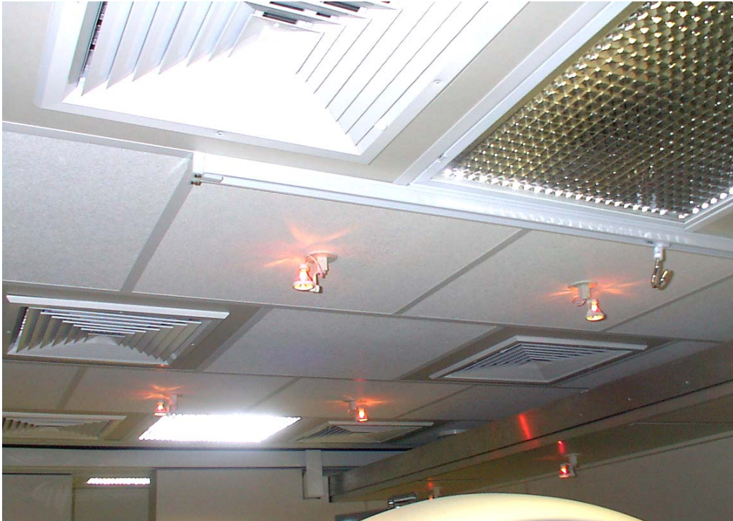
Figure 56: Gantry Room Overall Lighting
