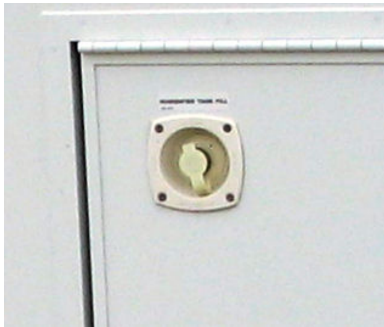
Figure 29: Humidifier Tank Fill
