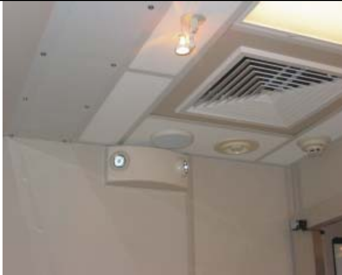
HVAC Vents Discharge
