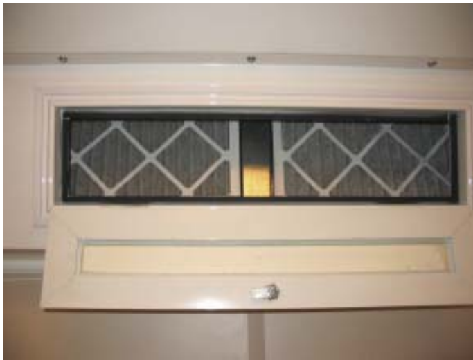
HVAC Filter Access
