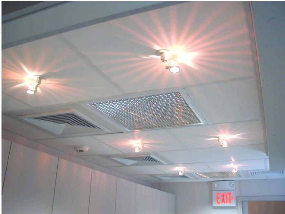
Figure 55: Control Room Overall Lighting
