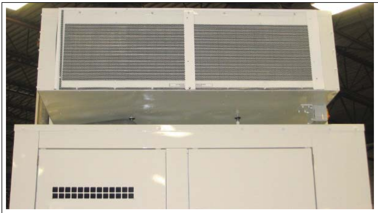
Figure 38: Northern Air A/C Units
