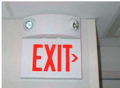
Control Room Emergency Light
