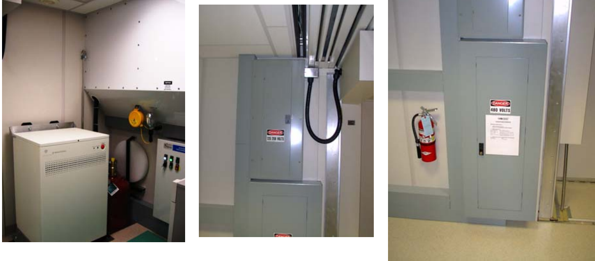
Figure 30: 480V and 120/208V AC Electrical Panels
