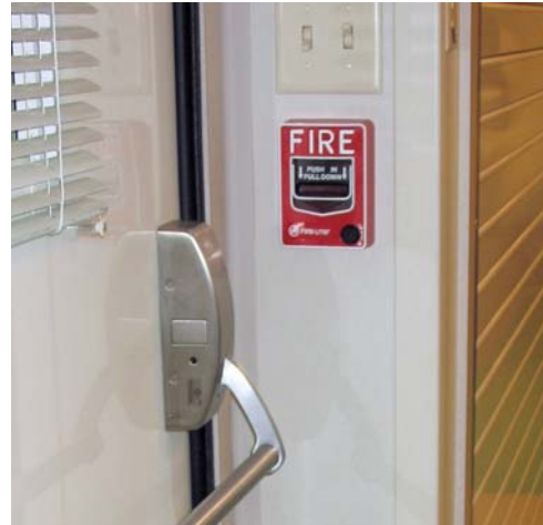
Figure 20: Fire Alarm Pull Station
