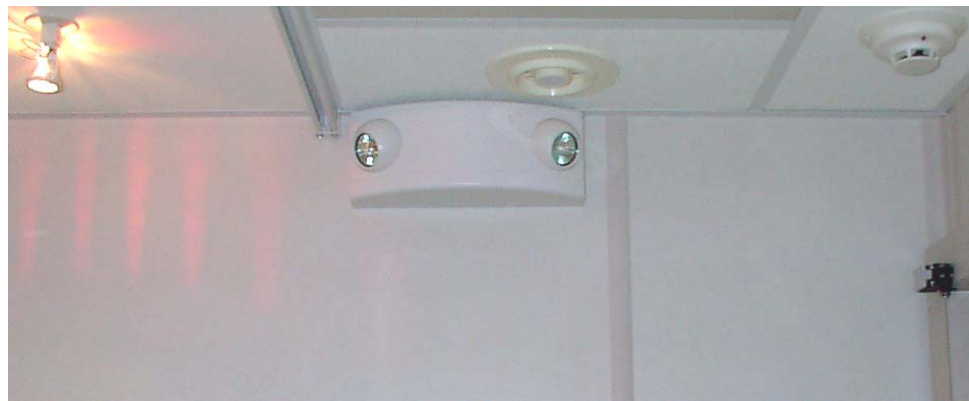
Dispensing Room Emergency Light
