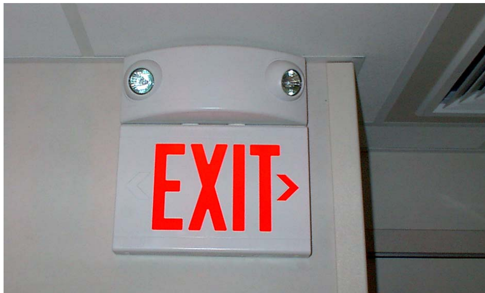
Figure 16: Control Room Exit & Emergency Lighting
