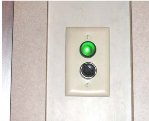
Figure 44: Platform Lift Power Switch
