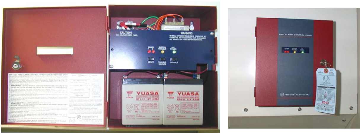
Figure 19: Fire Alarm Control Panel
