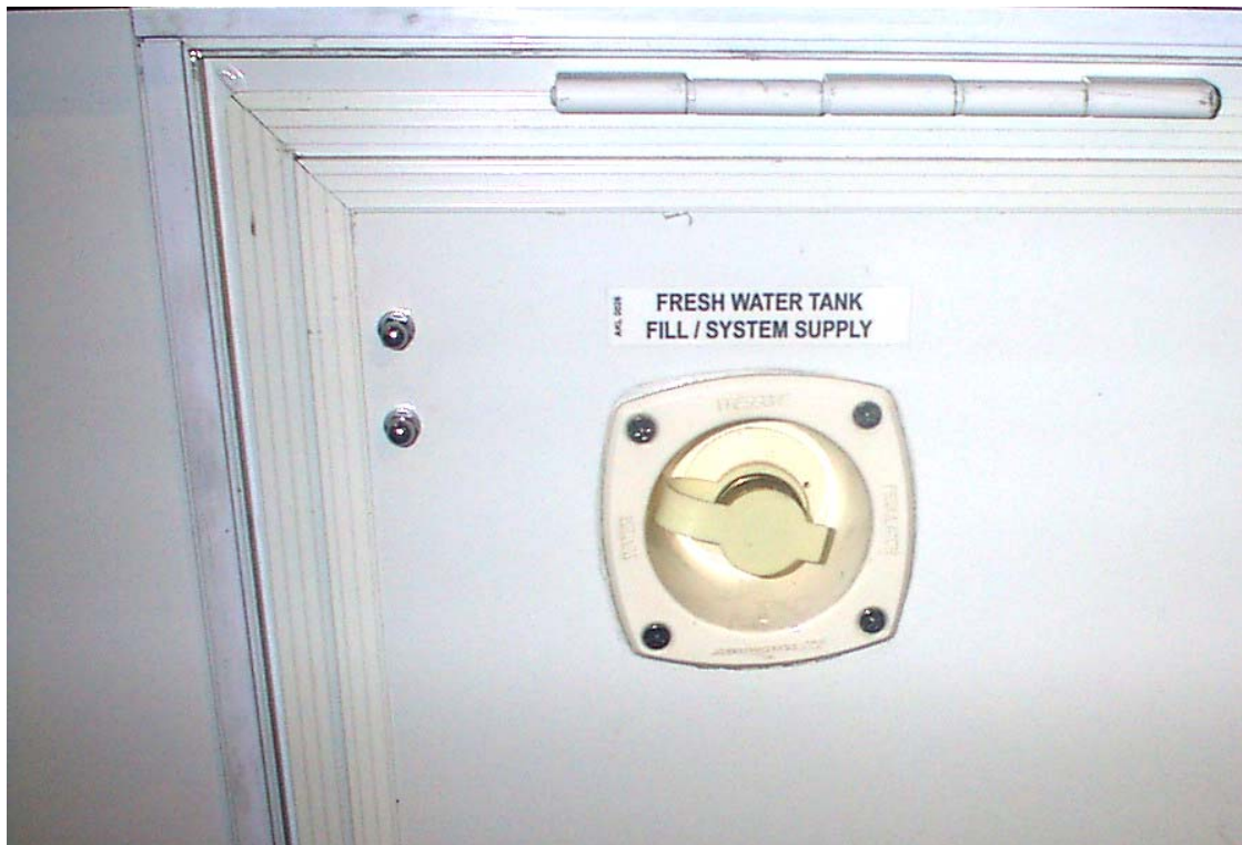
Figure 36: Fresh Water Connection
