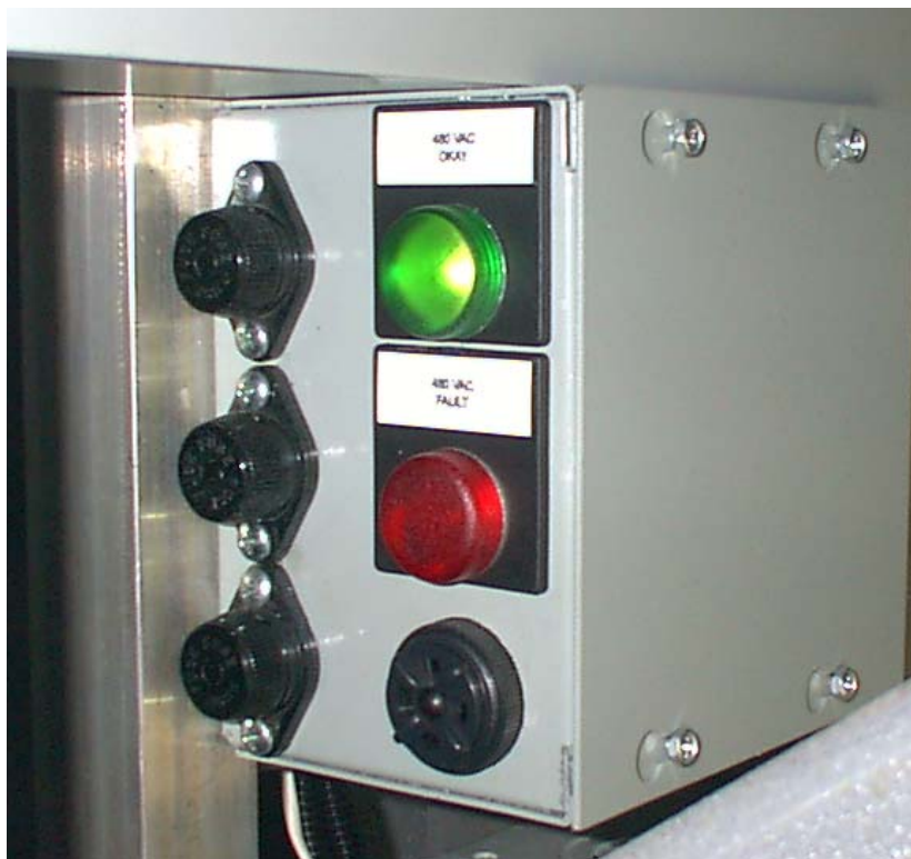
Figure 32: 480V AC Phase Power Monitor
