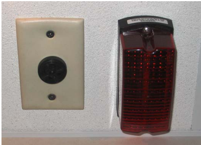
Figure 45: Platform Lift Strobe & Alarm
