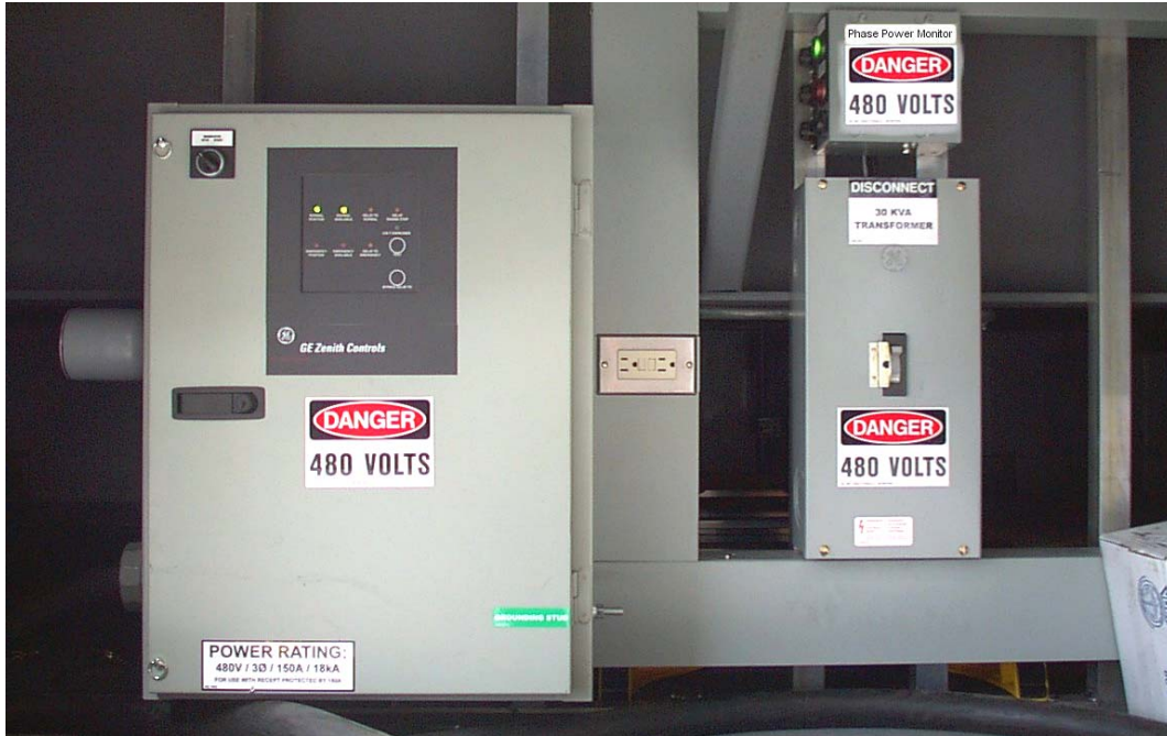
Figure 28: Automatic Transfer Switch and Phase Power Monitor
