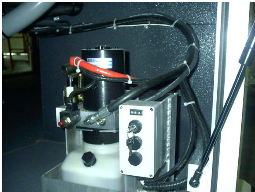
Figure 47: Platform Lift Service & Maintenance Controls
