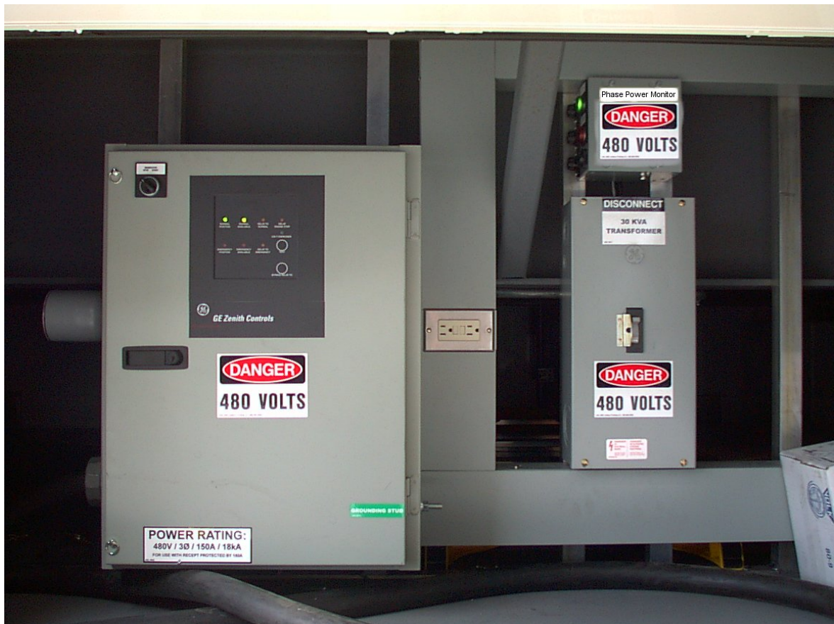
Figure 31: 480V AC ATS and Phase Power Monitor
