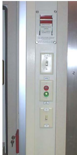
Figure 11 Mobile Unit Controls
